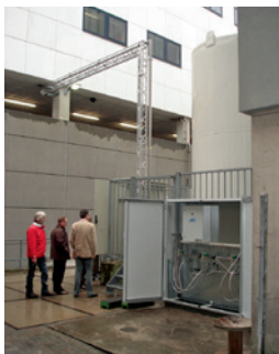
Filling station CryoMatic
